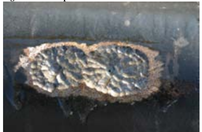
Figure 7: Close-up of External Corrosion with Pinhole
