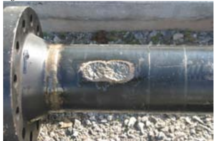
Figure 6: Overview of External Corrosion with Pinhole
